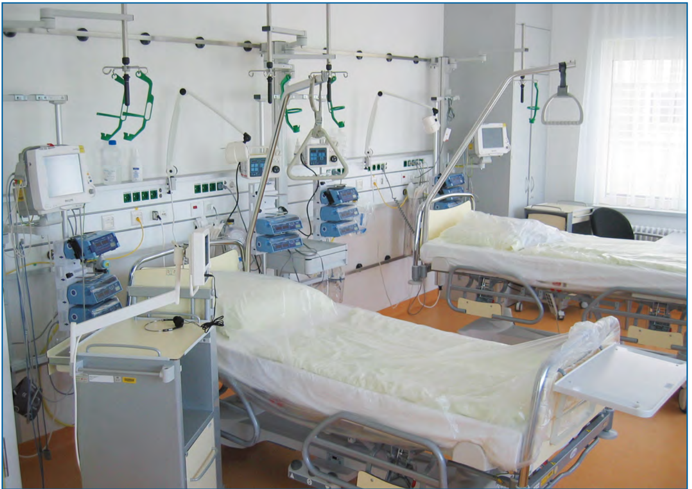
Fixing to wall supply duct and standard runner on the intensive-care station
