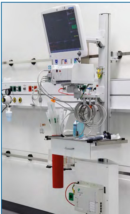
Fixing to wall supply duct and standard runner at the intensive-care station
